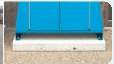
CONCRETE MOUNTING PAD
